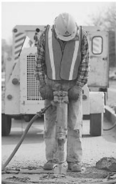
Figure 1. Repairs to utilities are a common sight in cities, incurring costs to cities and taxpayers.
