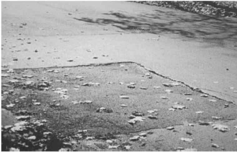
Figure 7. Pavement damage from settlement and shrinkage of cold patch asphalt.
